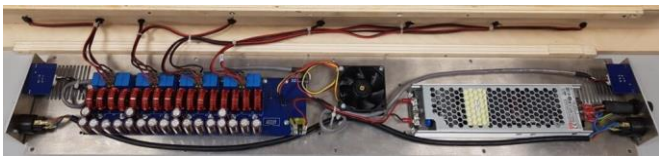
Figure 3 – Interiors of the electronics compartment.
